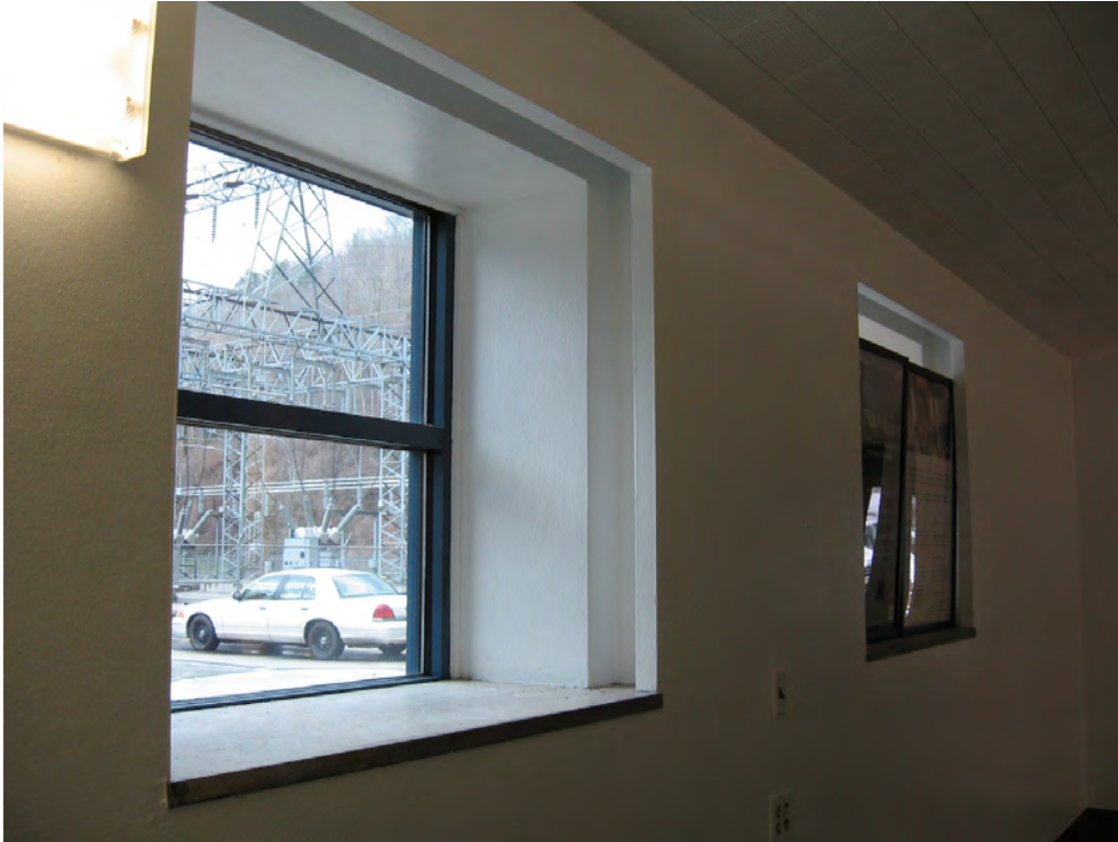
Figure 66: On the south elevation of the Control Room are two ca. 1990 fixed two-light aluminum sash windows. New steel mesh panels will be added behind these windows on the interior for increased security.
