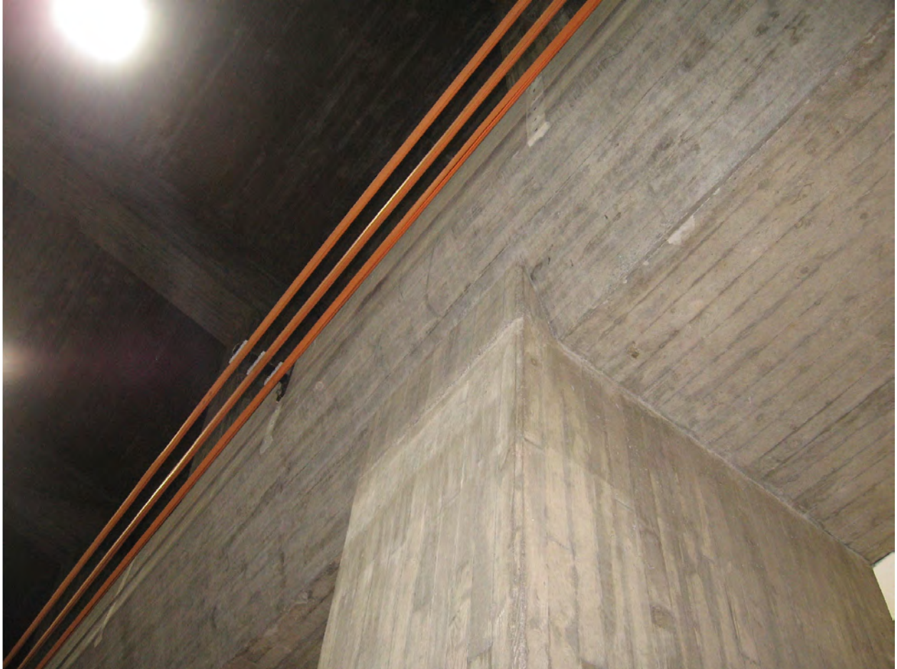
Figure 24: A new Avigilon security camera will be mounted just below the bottom railing for monitoring access to the double doors and the southwest entrance on the south elevation of the Turbine Floor.
