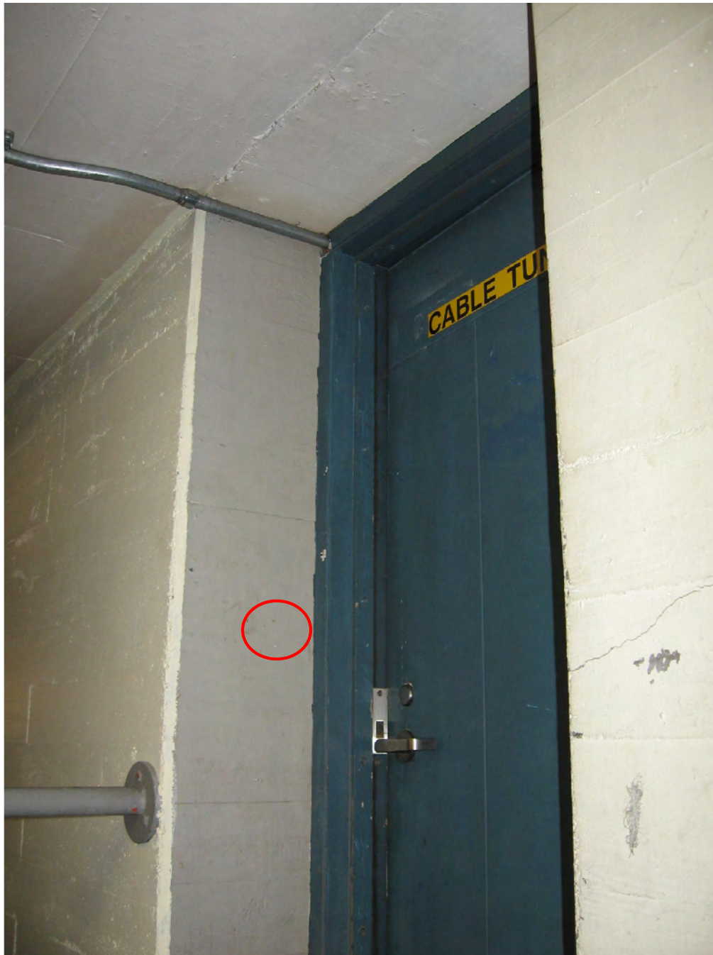
Figure 52: The red circle identifies the location of the card reader for the north Spreading Room Cable Tunnel door.
