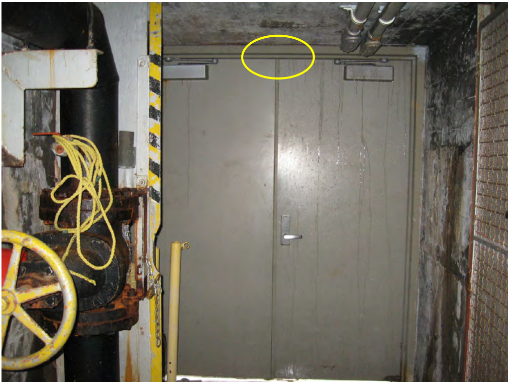
Figure 41: View is of the interior of the Head Gate Gallery doors. The location of the passive infrared sensor (PIR) is shown as the yellow circle.
