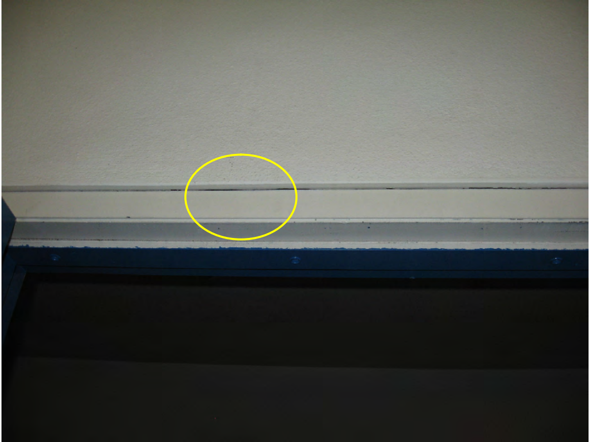
Figure 64: The location of the proposed PIR sensor is shown as the yellow circle on the interior of the Print Room door.
