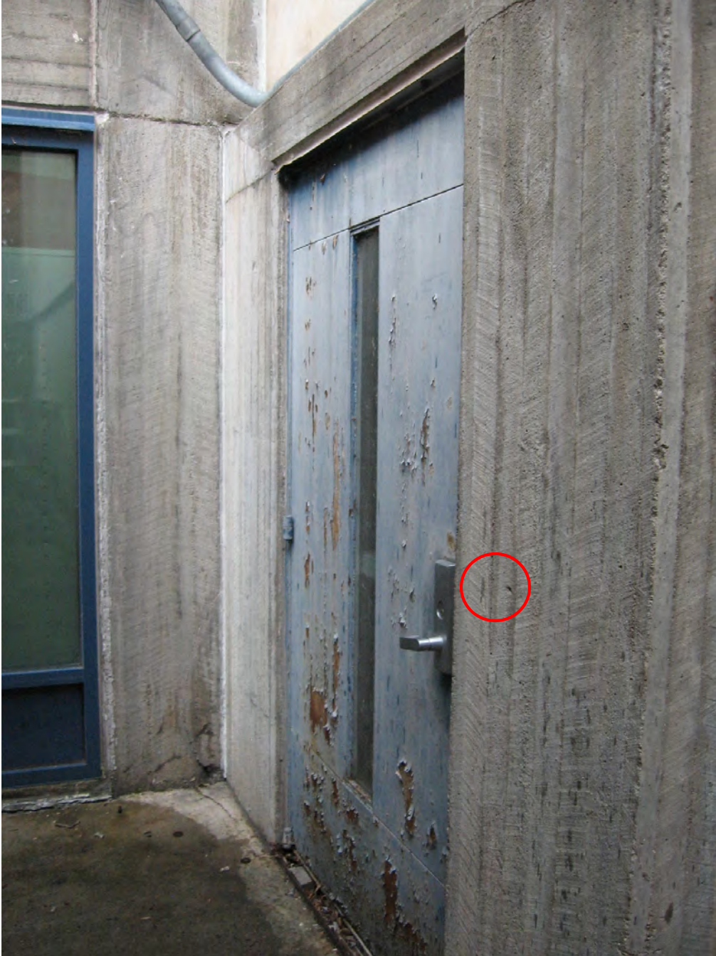
Figure 25: A security card reader will be added to this location circled in red adjacent to the northeast Powerhouse door.
