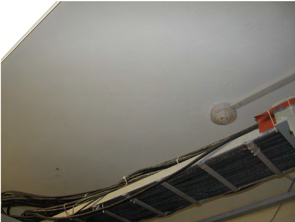
Figure 62: Ceiling location for the proposed Avigilon camera on the interior of the Communications Room south double doors.
