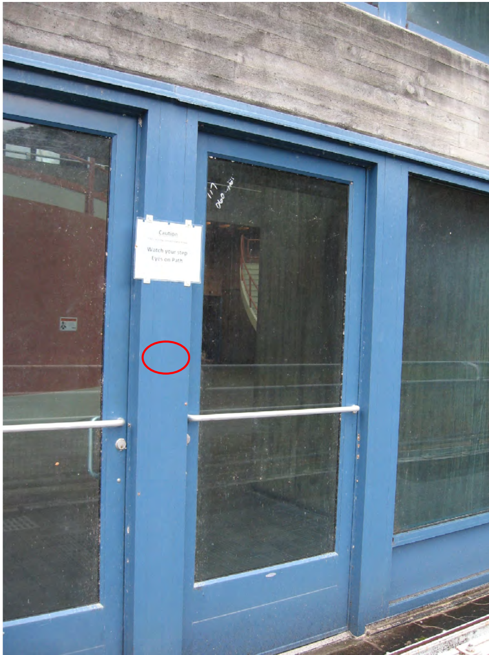
Figure 22: A security card reader will be added to this location circled in red adjacent to the double doors to the Turbine Floor on the south elevation of the powerhouse.
