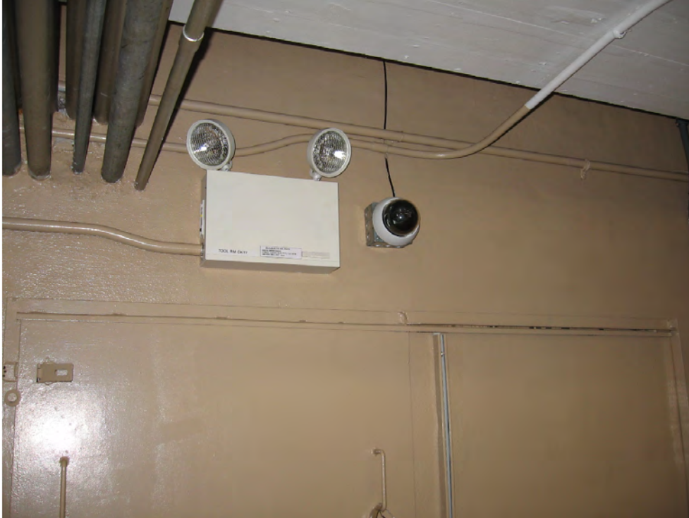
Figure 8: The new Avigilon security cameras to be installed in the powerhouse will be similar to this one in use at the Wilson Powerhouse in Alabama. This is a wall-mounted example.
