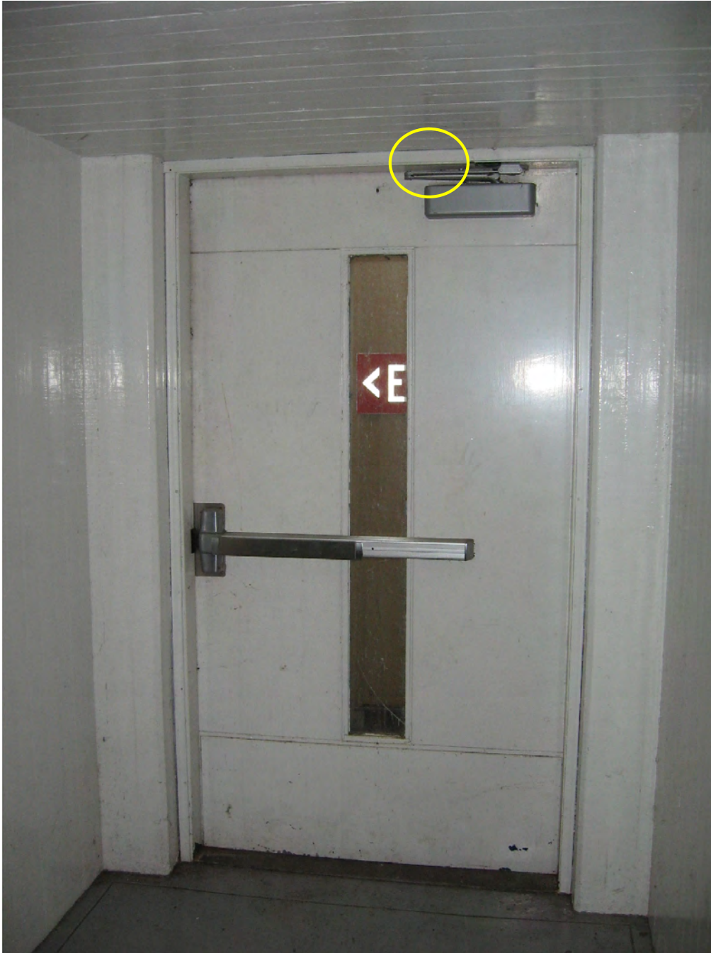
Figure 26: This view is of the interior of the northeast Powerhouse door. The location of the passive infrared sensor (PIR) is shown as the yellow circle.
