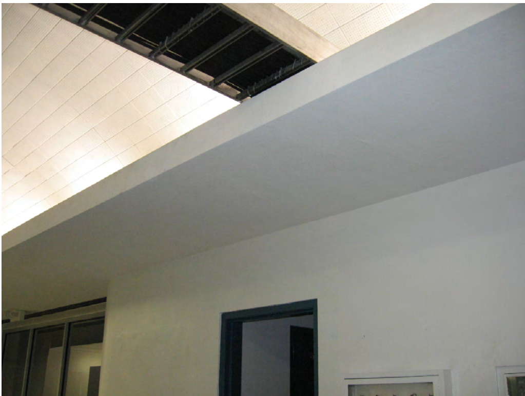
Figure 45: The new Avigilon camera will be placed along this section of the wall or ceiling to monitor the east Control Room door.
