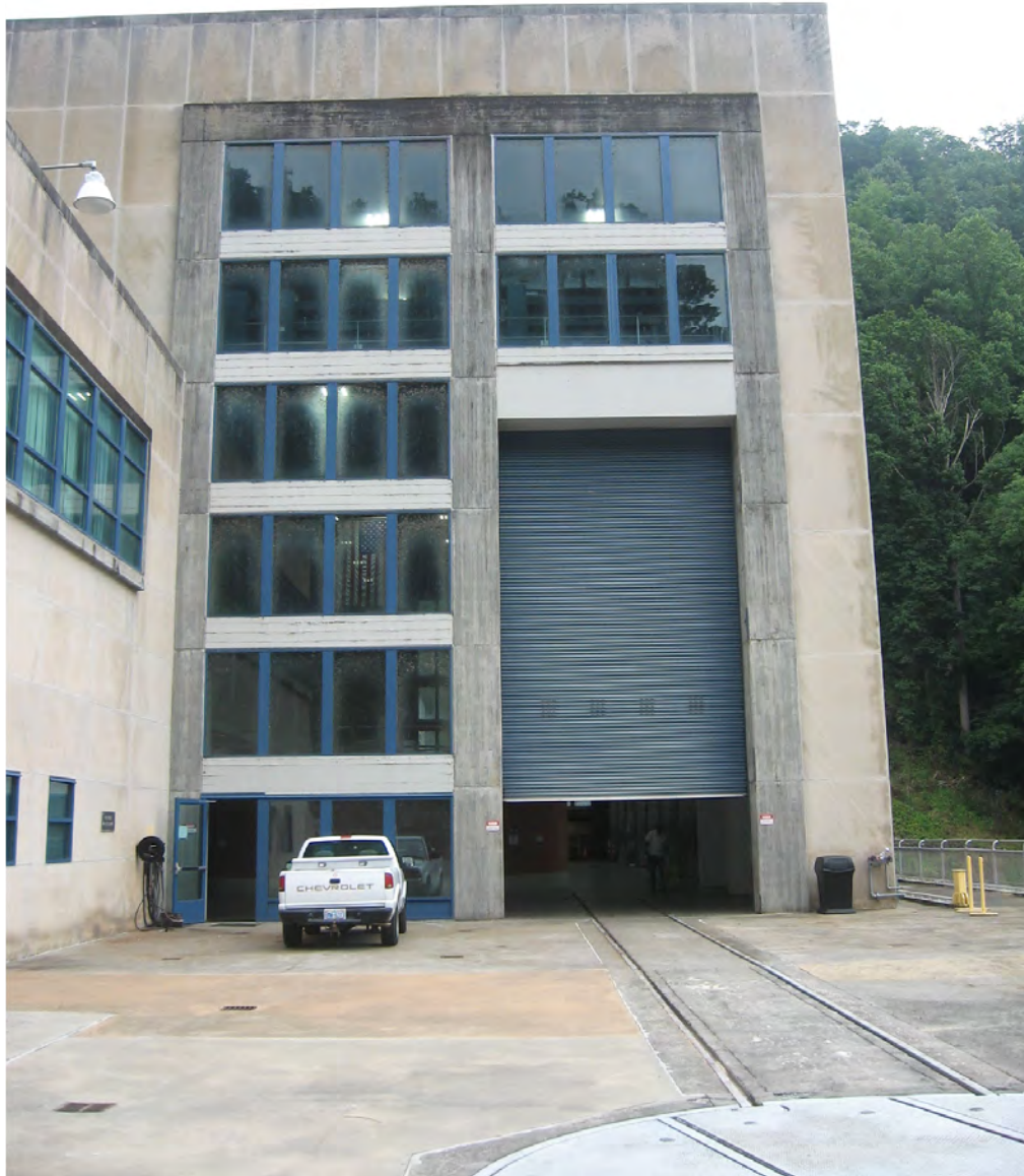
Figure 14: Primary entrance to the Fontana Powerhouse on the west elevation. This existing steel roll-up door was added ca. 2000.
