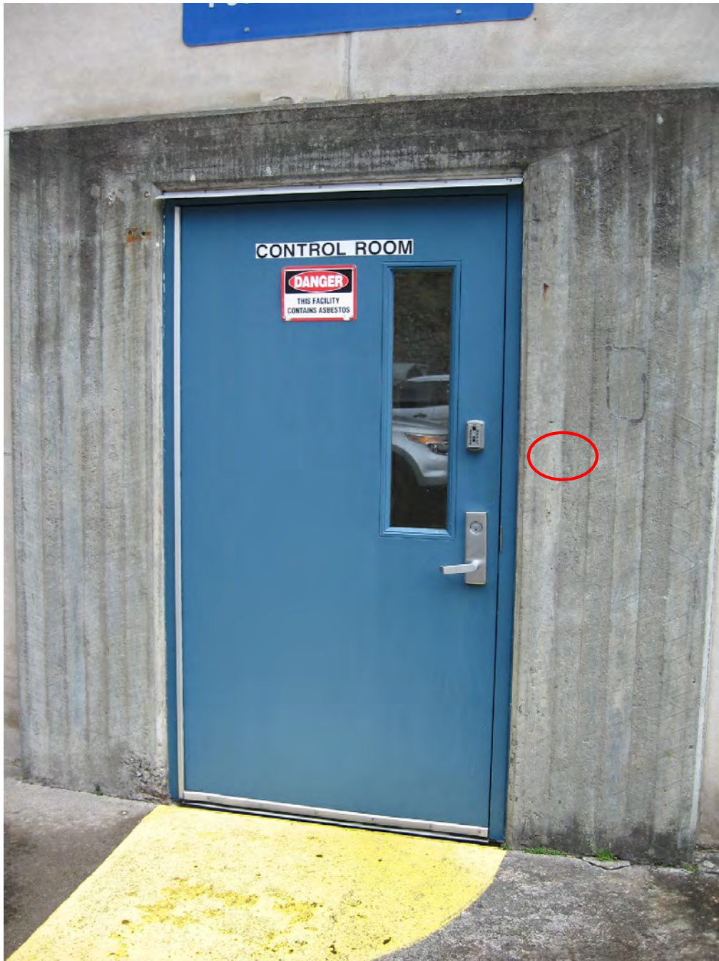
Figure 17: A security card reader will be added to this location circled in red at the southwest Control Room door of the powerhouse.
