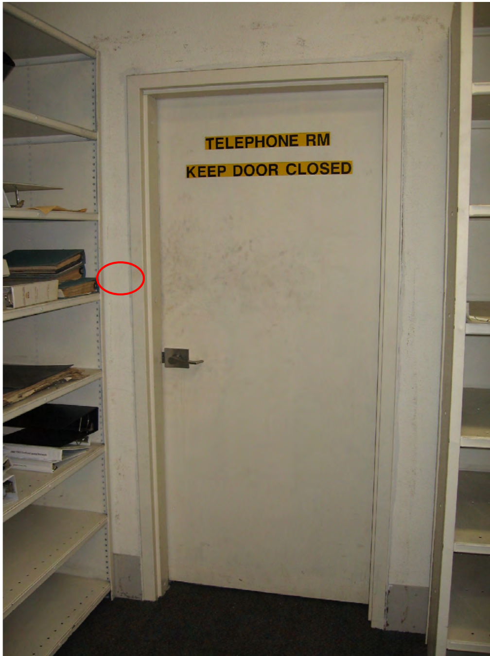
Figure 58: View of the Communications Room south door and the red circle shows the proposed location of the card reader.
