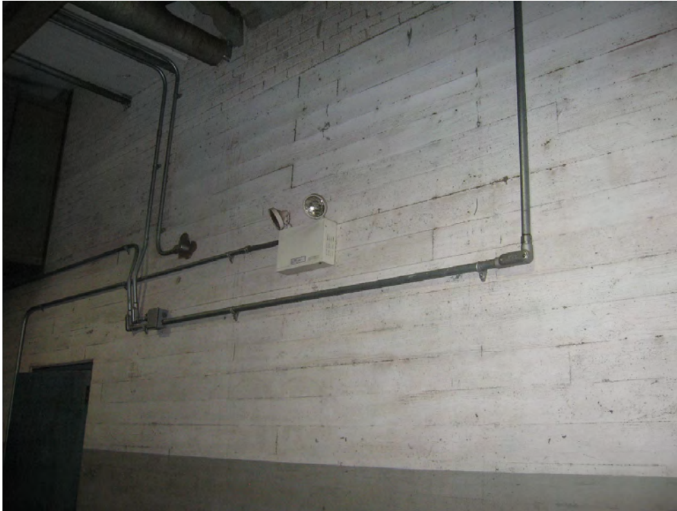
Figure 33: A new Avigilon security camera will be added along this wall inside the upper rear deck door. The wiring for this camera will follow the existing conduit as much as possible.
