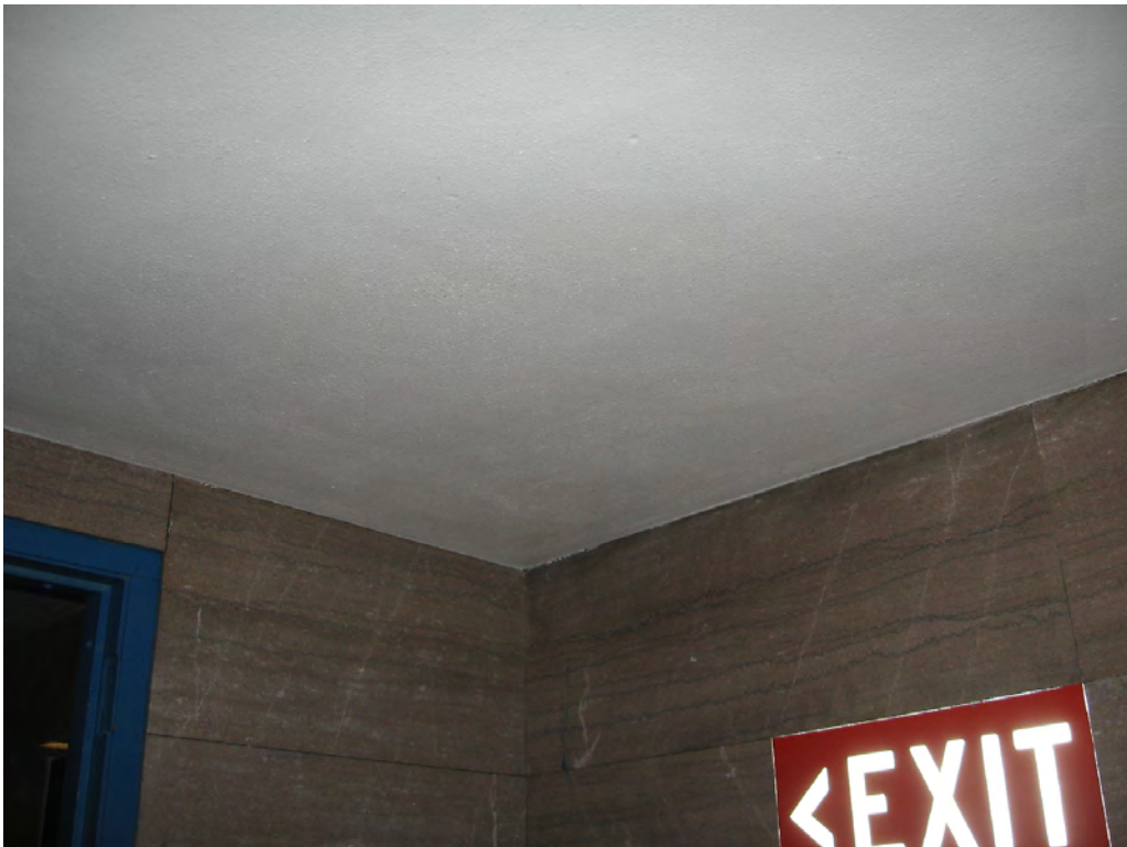
Figure 48: Ceiling location for the proposed Avigilon camera on the interior of the Incline Car Room door.
