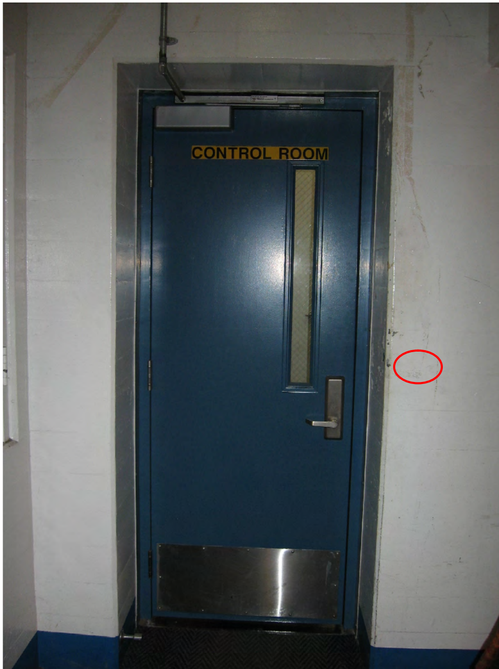
Figure 43: The east Control Room door will have a card reader installed at the location shown as the red circle.
