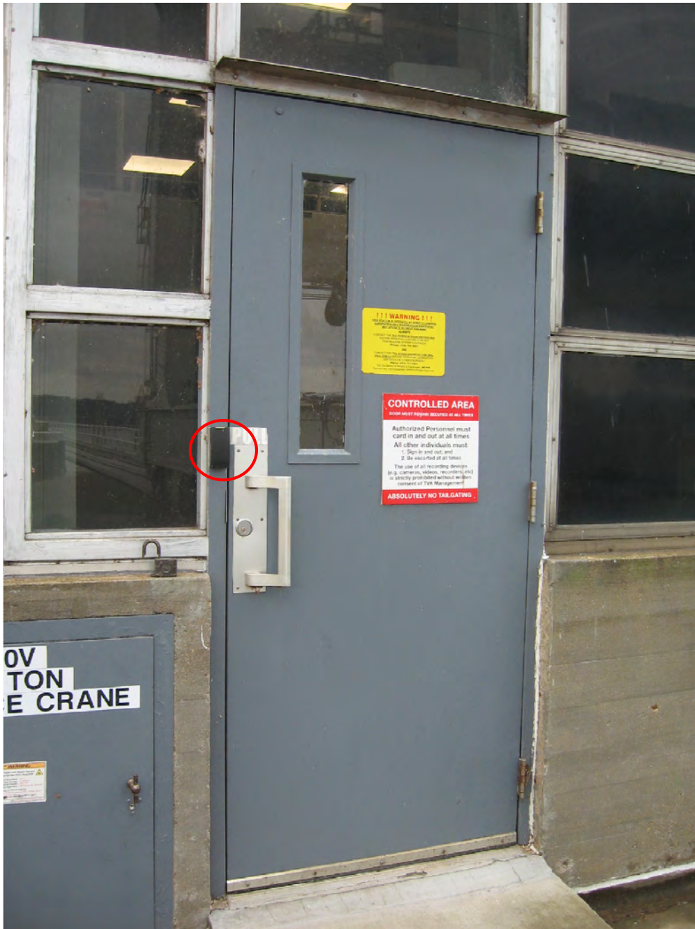
Figure 12: On the exterior of the door the PIR sensor will not be visible. The new exterior security card readers to be installed in the powerhouse will be similar to this one in use at the Wheeler Powerhouse in Alabama. The red circle shows the card reader location.
