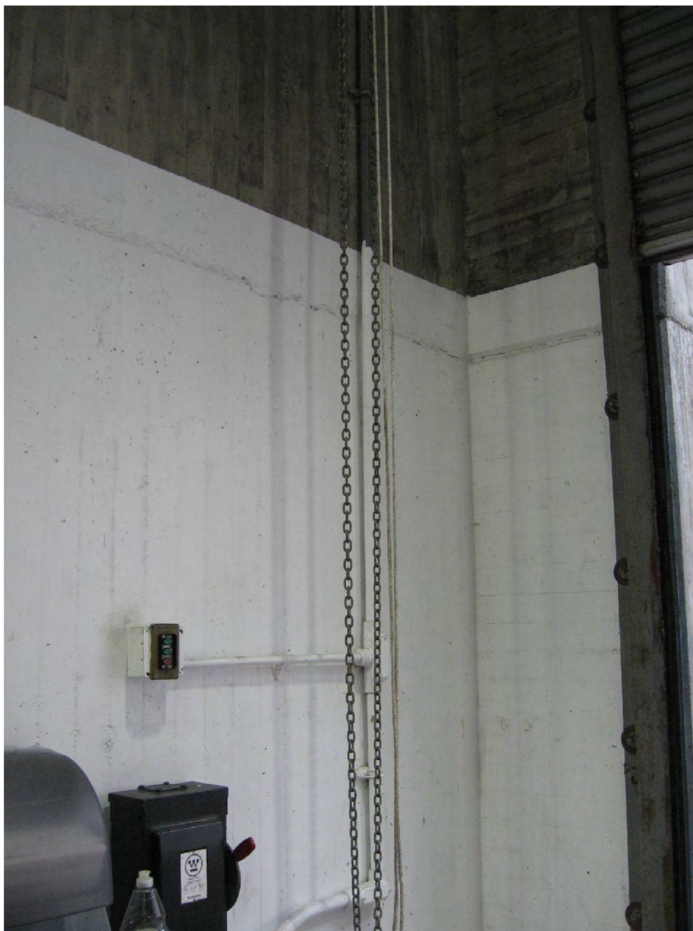
Figure 16: A new Avigilon security camera will be added to this wall and the wiring will utilize the existing conduit as much as possible.
