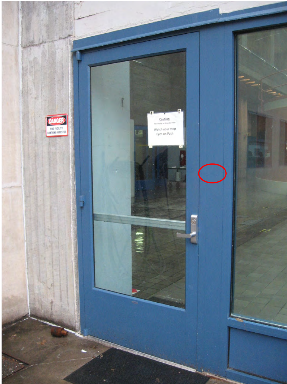
Figure 20: A security card reader will be added to this location circled in red adjacent to the southwest entrance to the Turbine Floor on the south elevation of the powerhouse.
