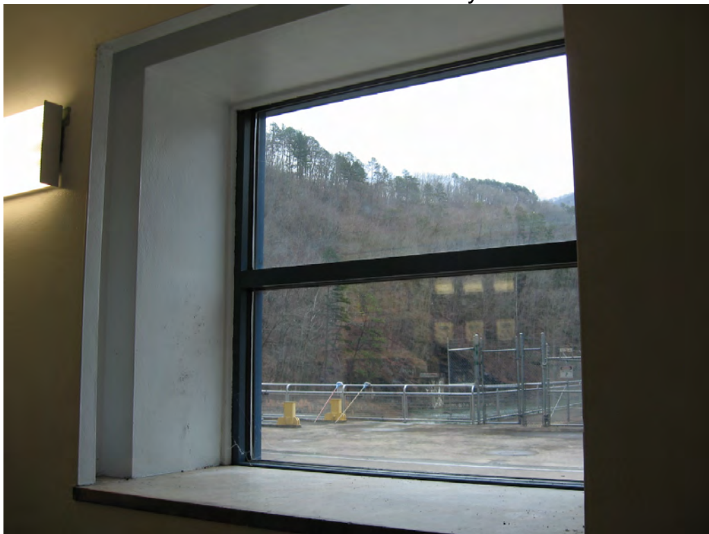
Figure 67: Detail of the Control Room's ca. 1990 fixed, two-light aluminum sash window. A new steel mesh panel will be added on the inside of the window.
