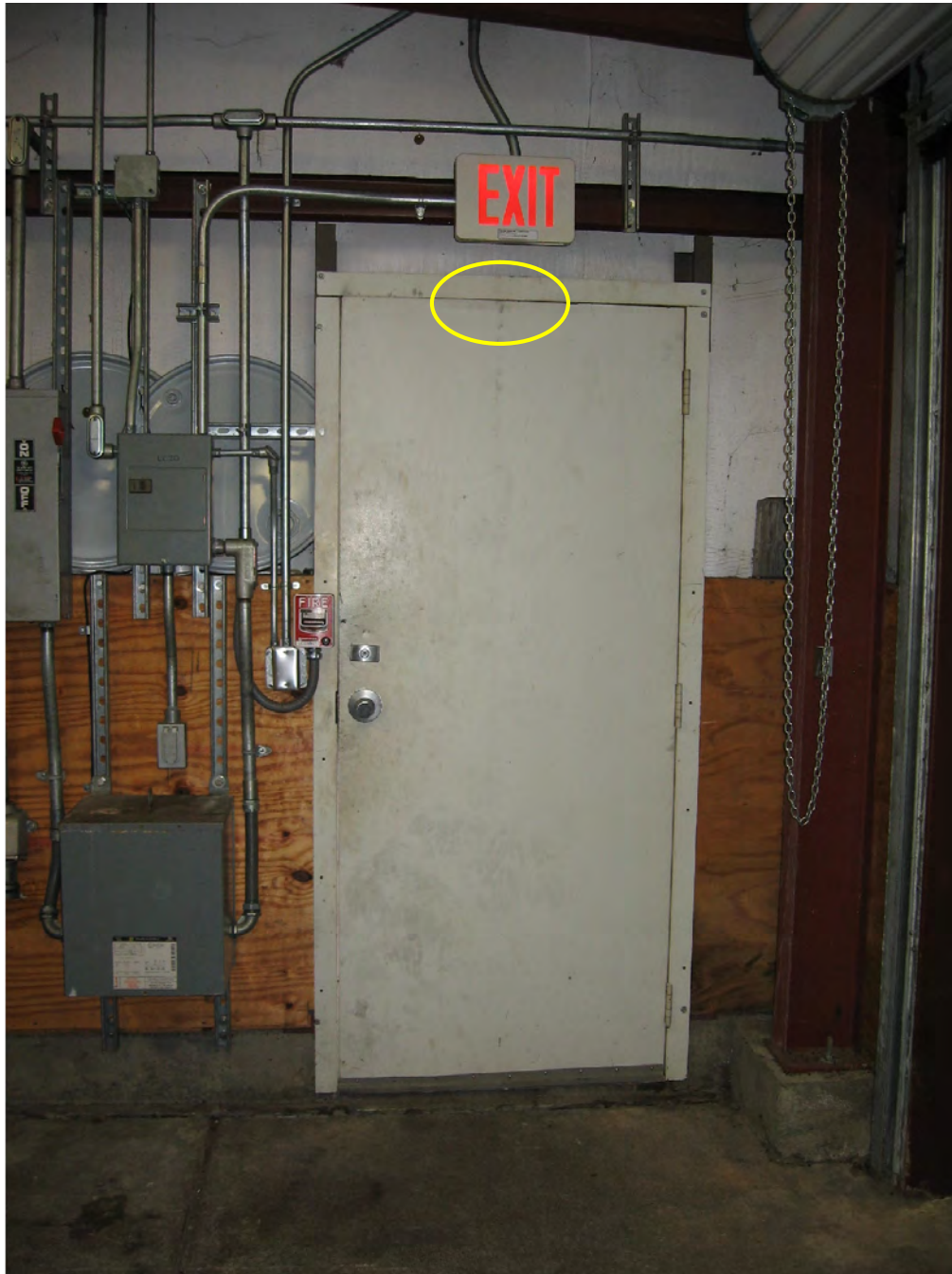
Figure 35: This view is of the interior of the Kelly Building door on the south elevation. The location of the passive infrared sensor (PIR) is shown as the yellow circle.
