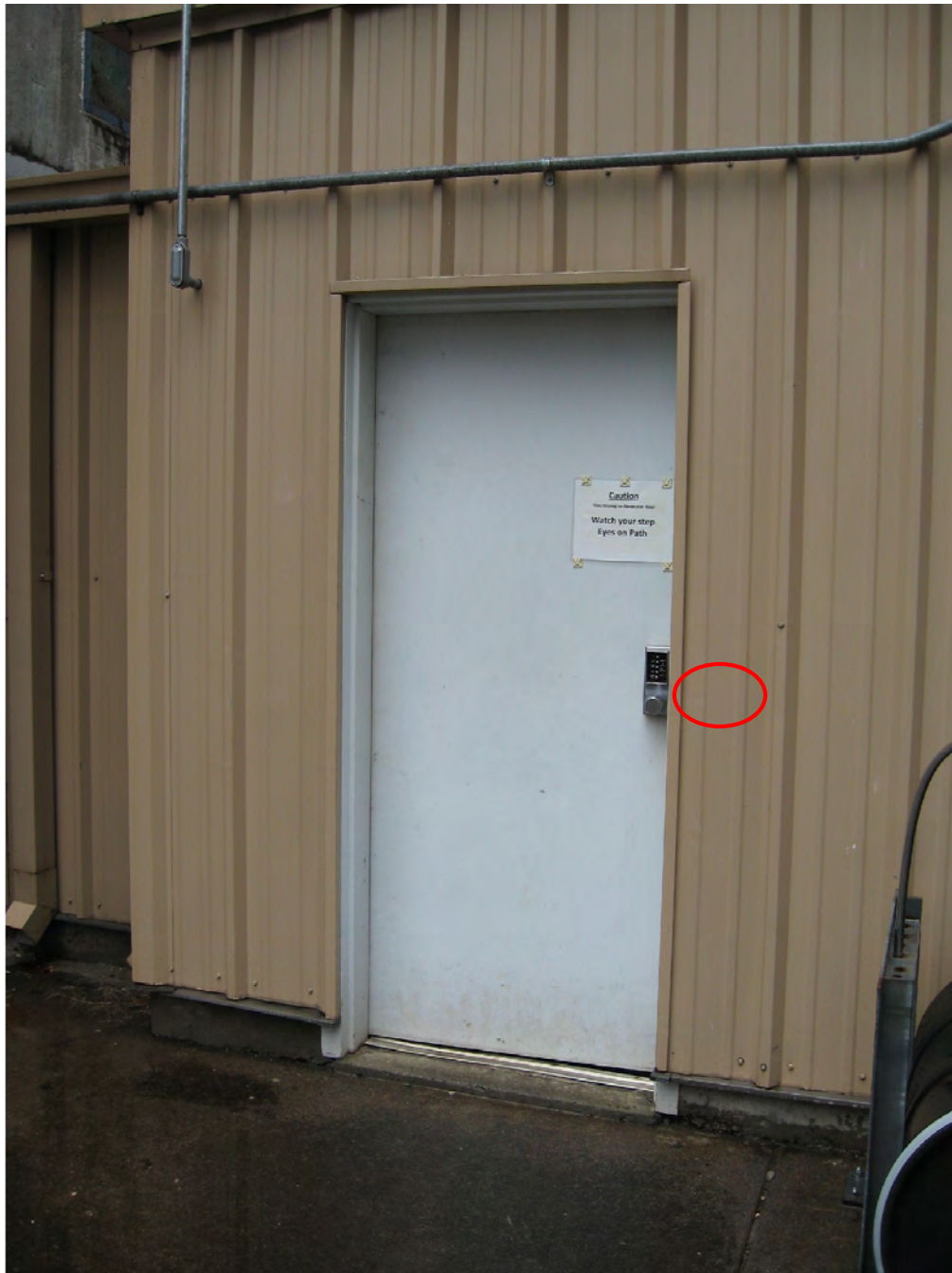
Figure 34: The Kelly Building is a small metal wing added ca. 1990 on the east elevation of the powerhouse. A card reader will be added to this entrance on the south elevation of the building. This card reader location is circled in red.
