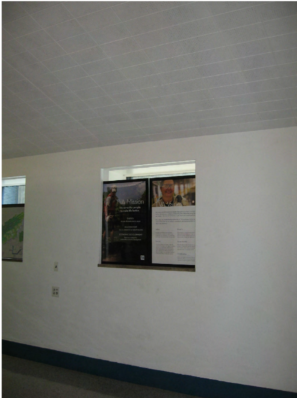
Figure 19: A new Avigilon security camera will be mounted at either the ceiling or wall at this location just inside the southwest Control Room door.
