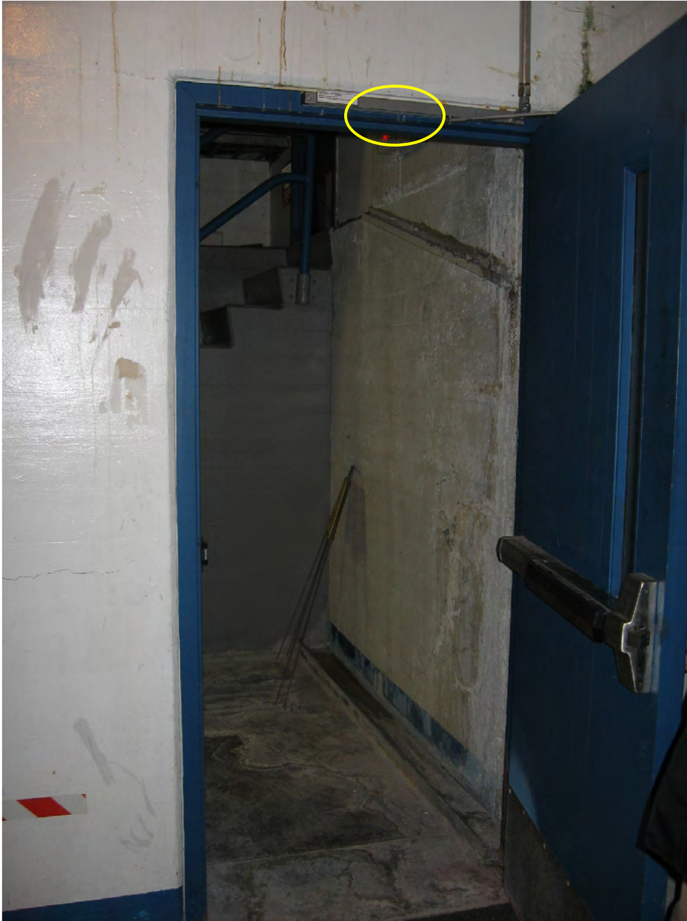
Figure 50: The location of the proposed PIR sensor on the interior of the northeast Spreading Room door is shown as the yellow circle.
