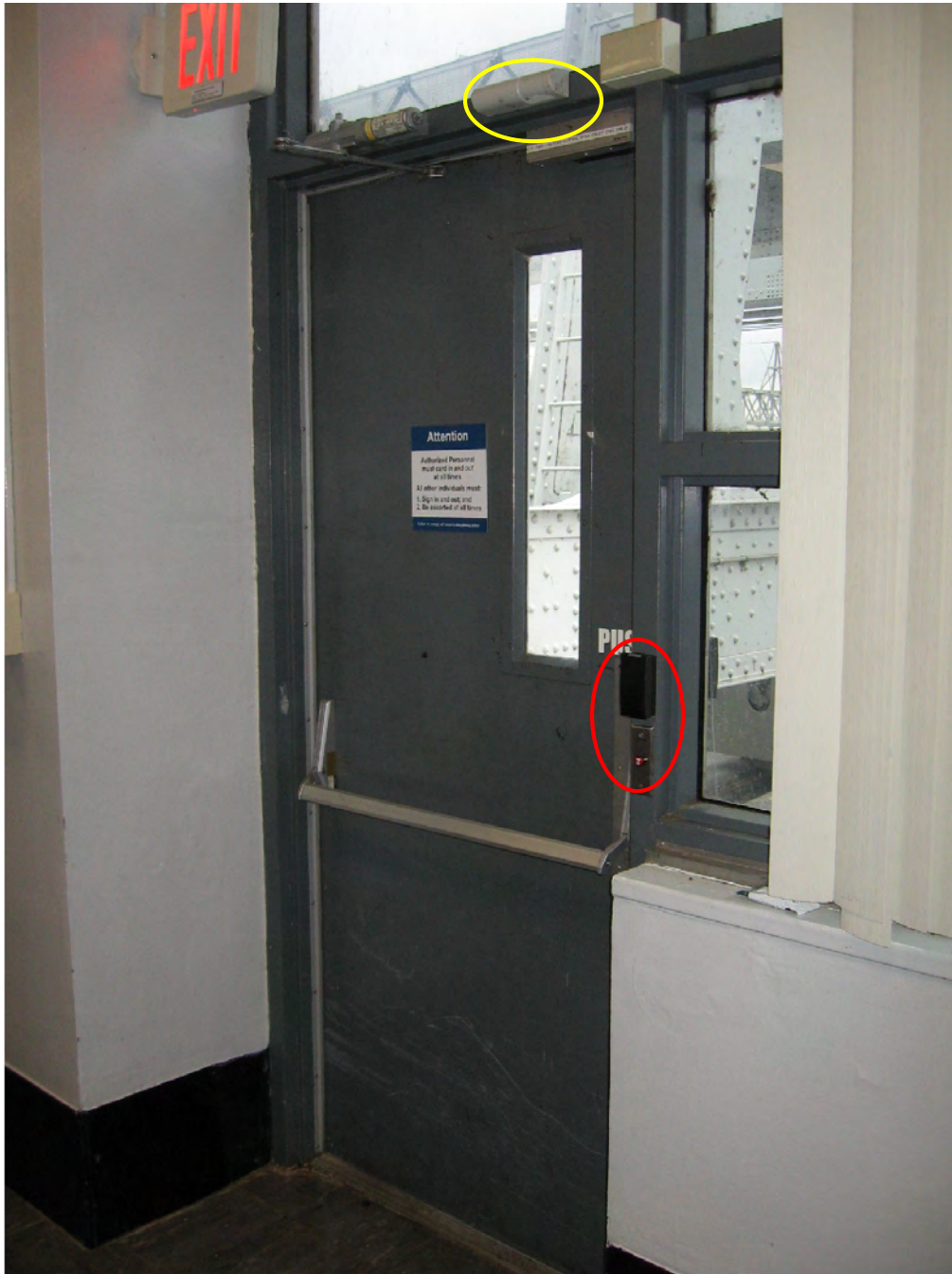
Figure 10: The new passive infrared (PIR) sensors and security card readers to be installed in the powerhouse will be similar to these at the Wheeler Powerhouse in Alabama. The red circle shows the card reader with a push button shunt and the yellow circle shows the PIR sensor.
