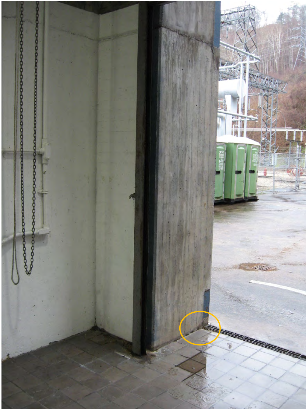
Figure 15: This view shows the interior of the roll-up door and the location of the floor mounted alarm contact is circled in orange.
