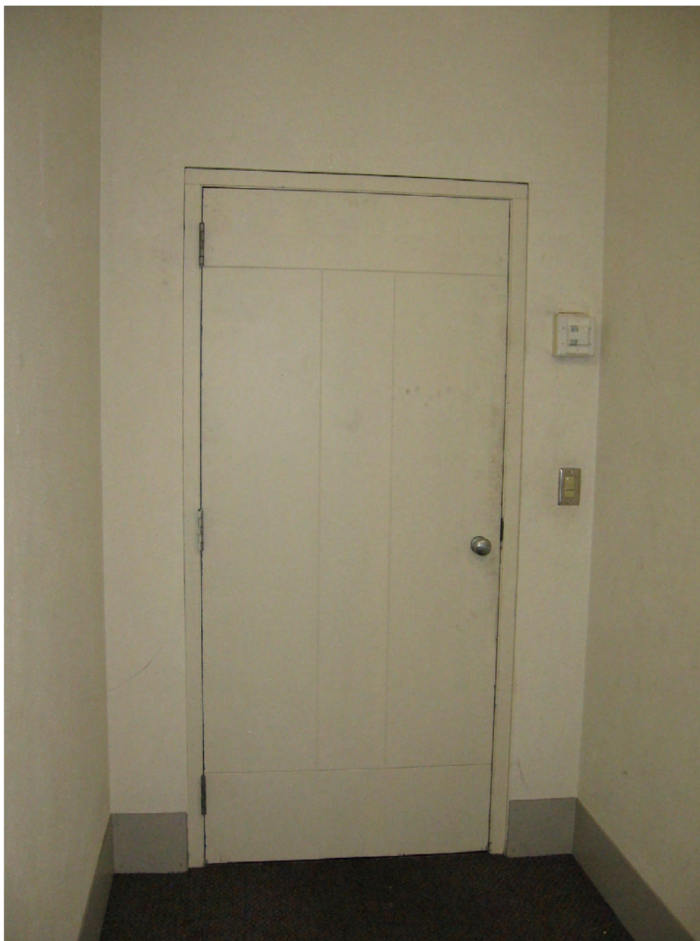
Figure 65: The location for the proposed Avigilon camera on the interior of the Print Room door will either be mounted at the ceiling or along the wall on the interior of the door.
