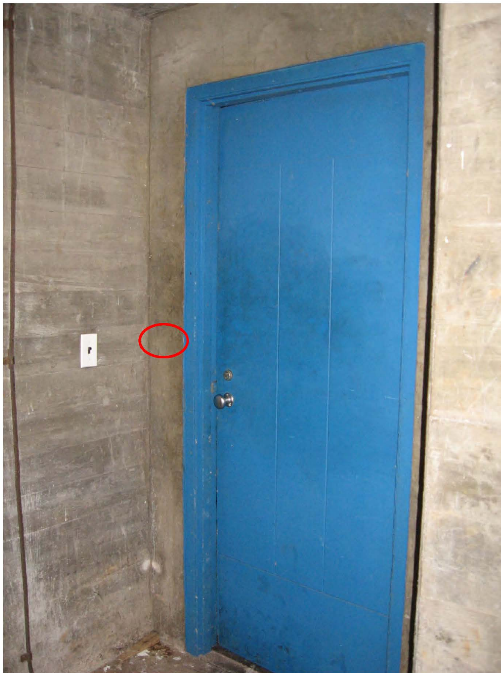
Figure 46: View of the Incline Car Room door with the red circle showing the location of the proposed card reader.
