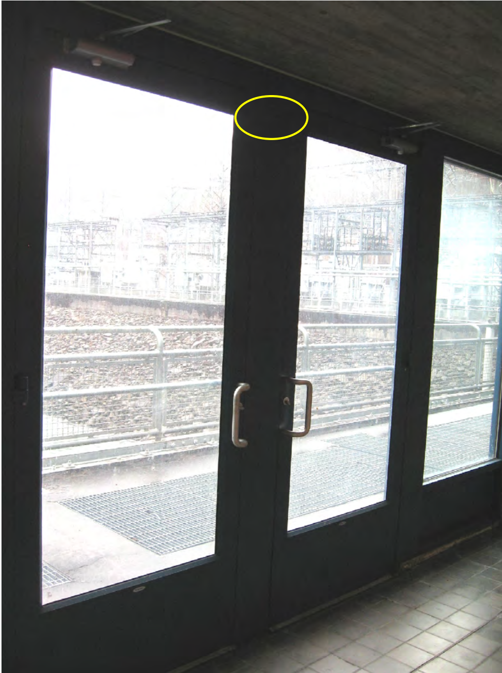
Figure 23: This view is of the interior of the double doors leading to the south elevation from the Turbine Floor. The location of the passive infrared sensor (PIR) is shown as the yellow circle.
