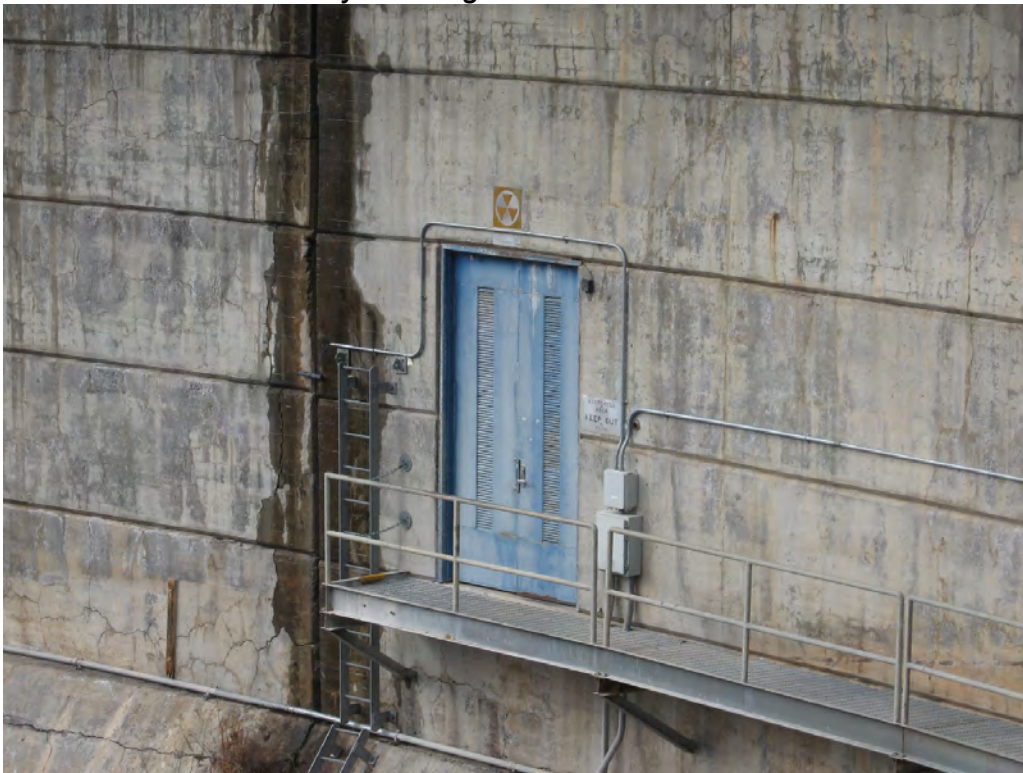
Figure 37: On the south face of the dam is the east-end Head Gate Gallery door. A card reader will be added to this entrance.
