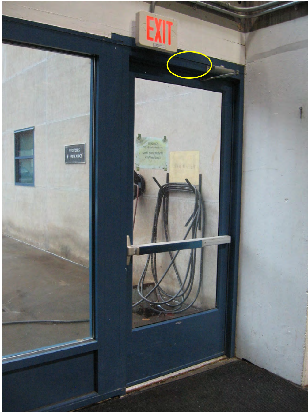
Figure 21: This view is of the interior of the southwest entrance to the Turbine Floor on the south elevation. The location of the passive infrared sensor (PIR) is shown as the yellow circle.
