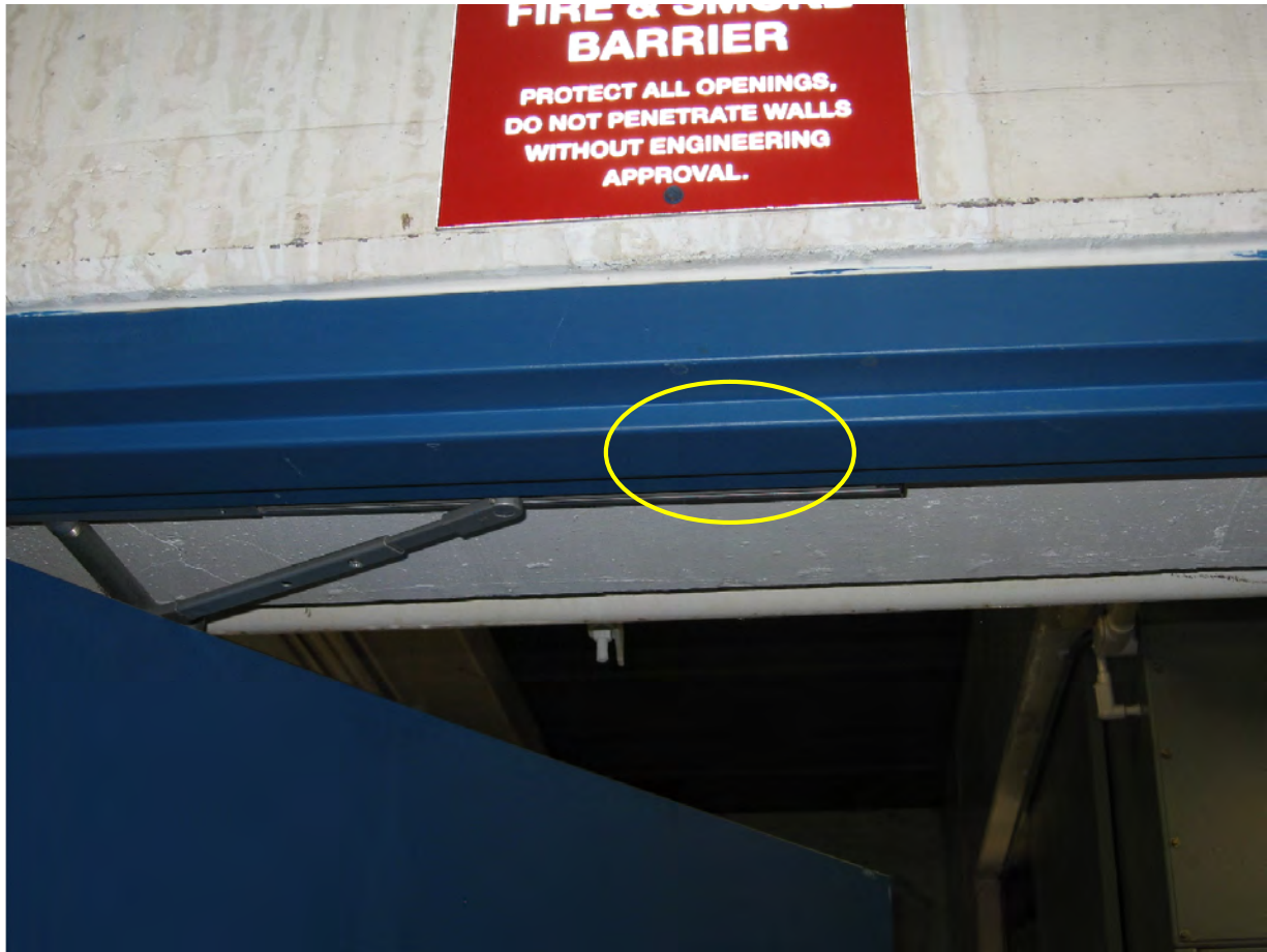
Figure 56: Location of the proposed PIR sensor on the interior of the southeast Spreading Room door.
