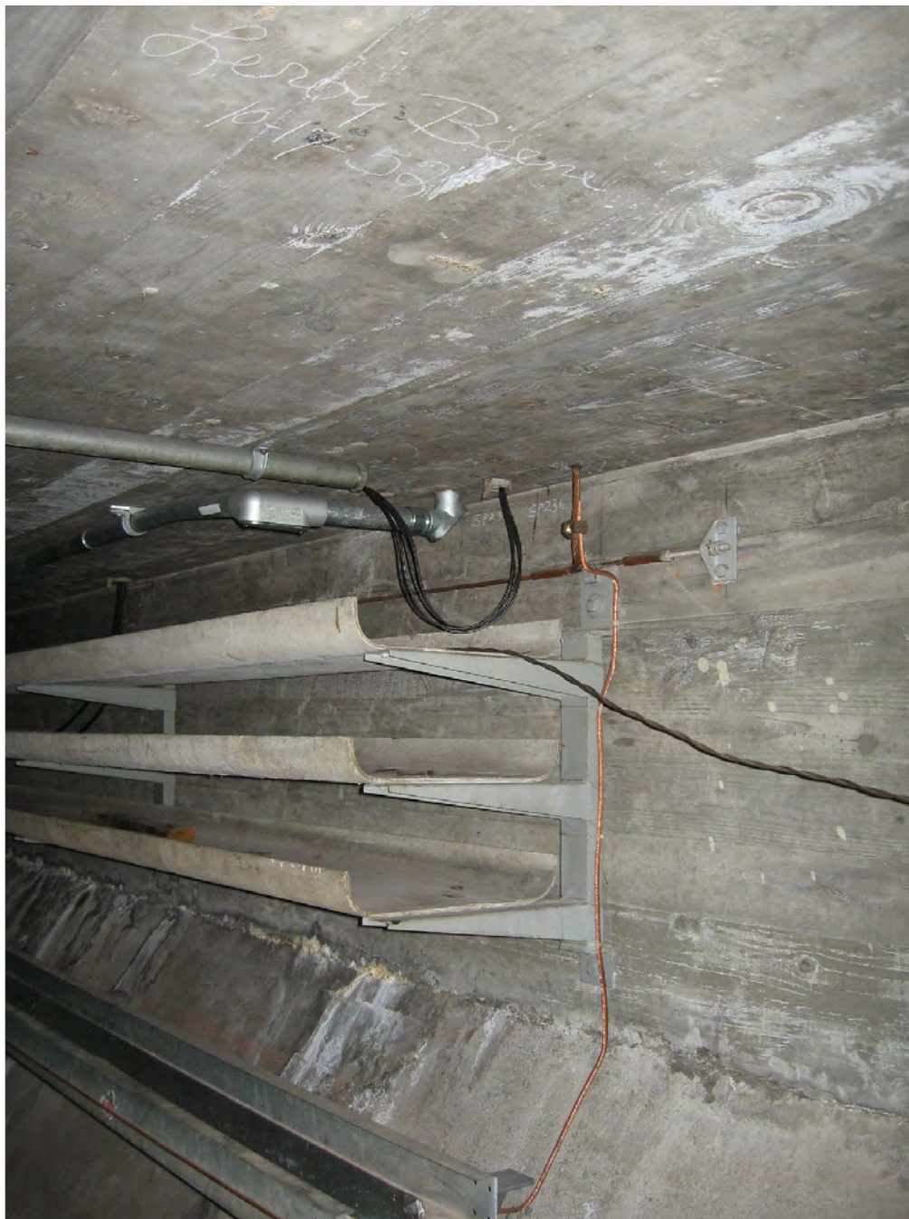
Figure 54: The location for the proposed Avigilon camera would be on the wall or ceiling of the interior of the cable tunnel behind the north Spreading Room Cable Tunnel door.
