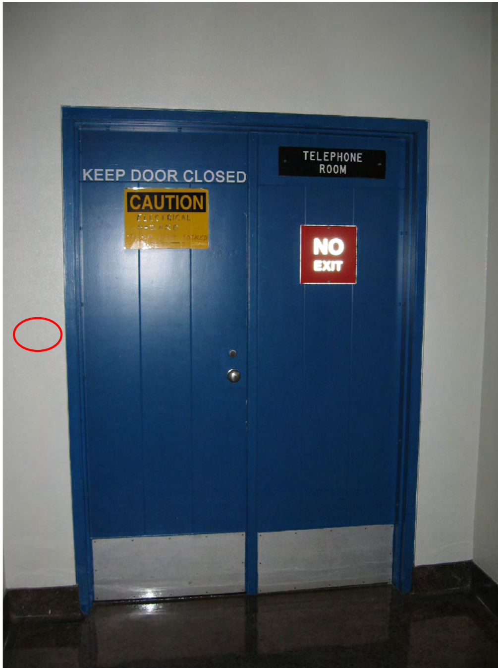
Figure 60: View of the Communications Room south double doors and the red circle shows the proposed location of the card reader.
