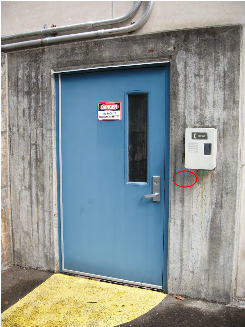
Figure 28: A security card reader will be added to this location circled in red adjacent to the northwest Powerhouse door.
