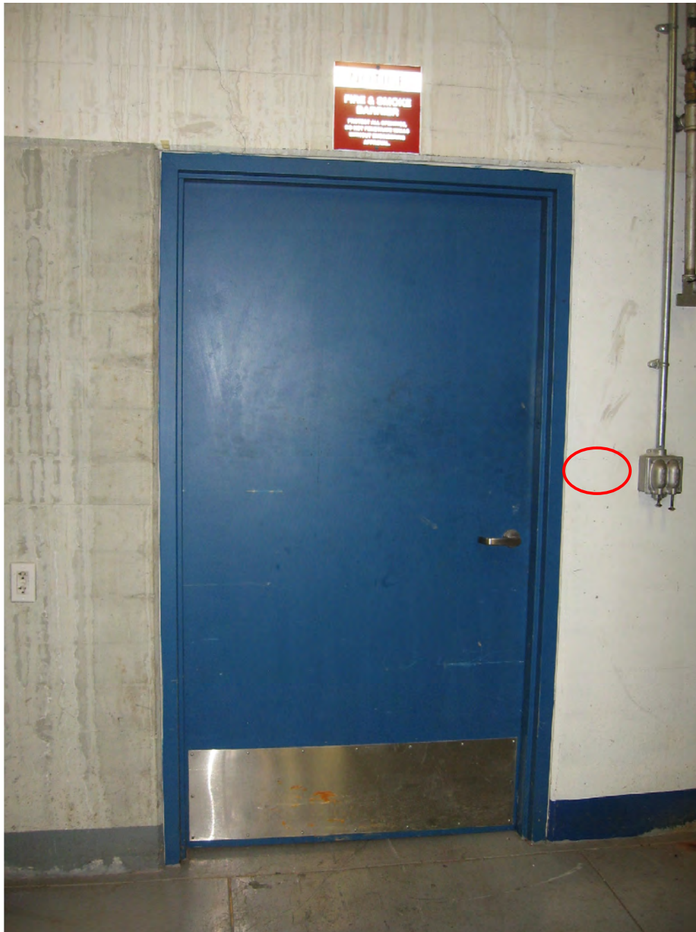
Figure 55: The red circle identifies the location of the card reader for the southeast Spreading Room door.
