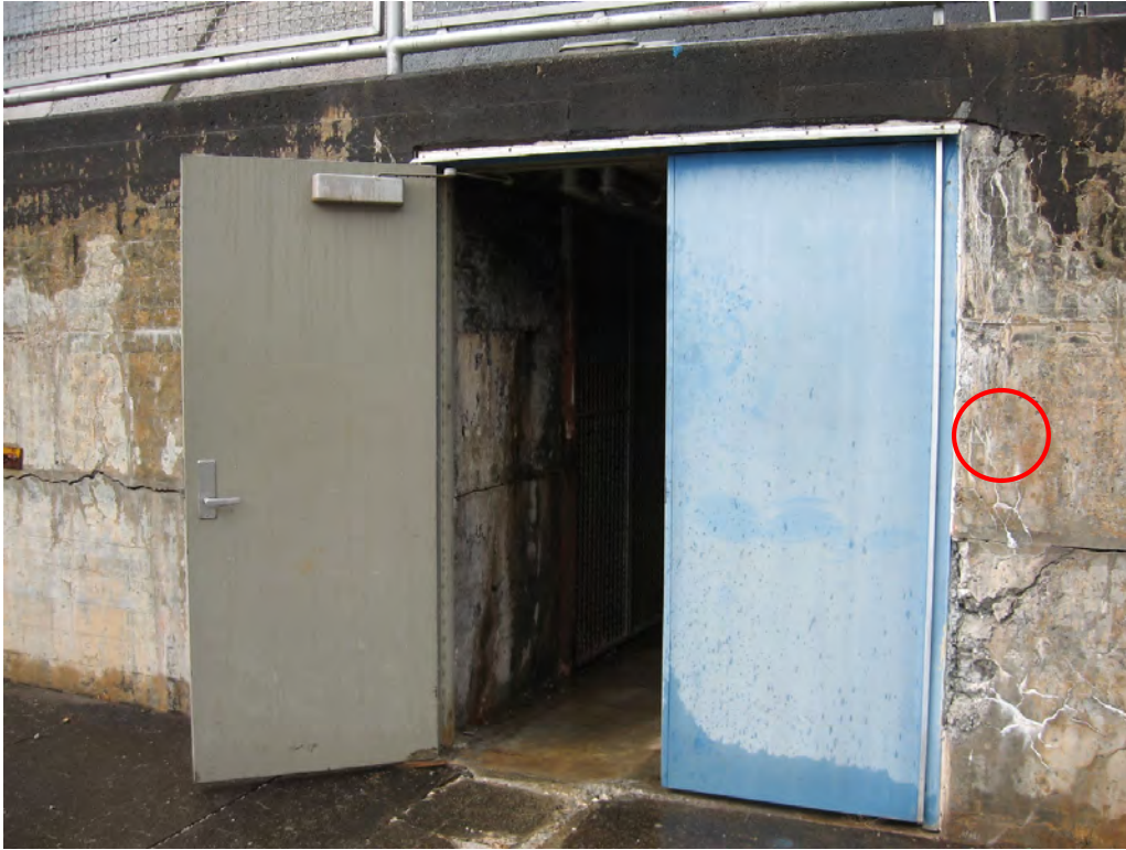
Figure 40: The Head Gate Gallery double doors are located on the south elevation of the dam. A new card reader will be added at the location shown circled in red.
