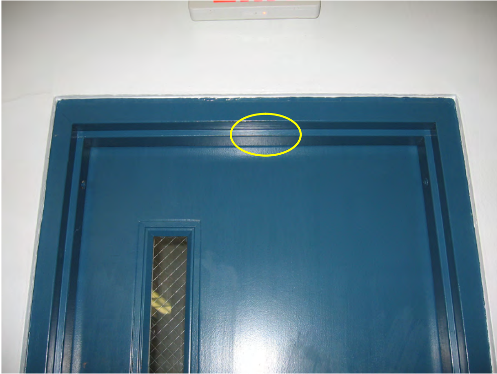
Figure 44: Interior of the east Control Room door showing the proposed location of the PIR sensor.
