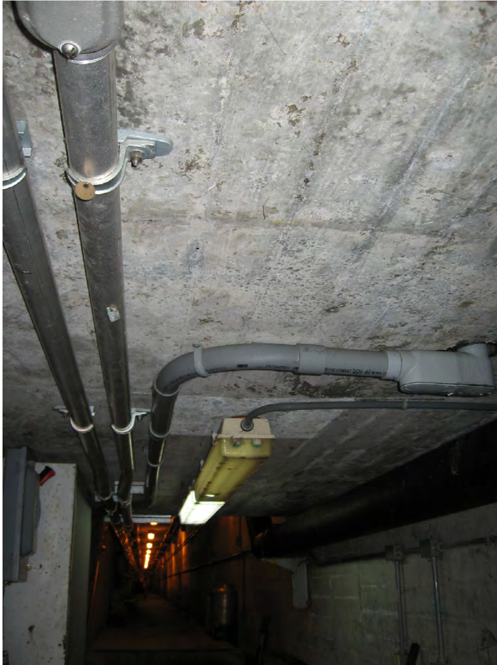
Figure 42: A new Avigilon security camera will be installed on the ceiling just inside the Head Gate Gallery double doors. The wires will be run along the existing conduits as much as possible.
