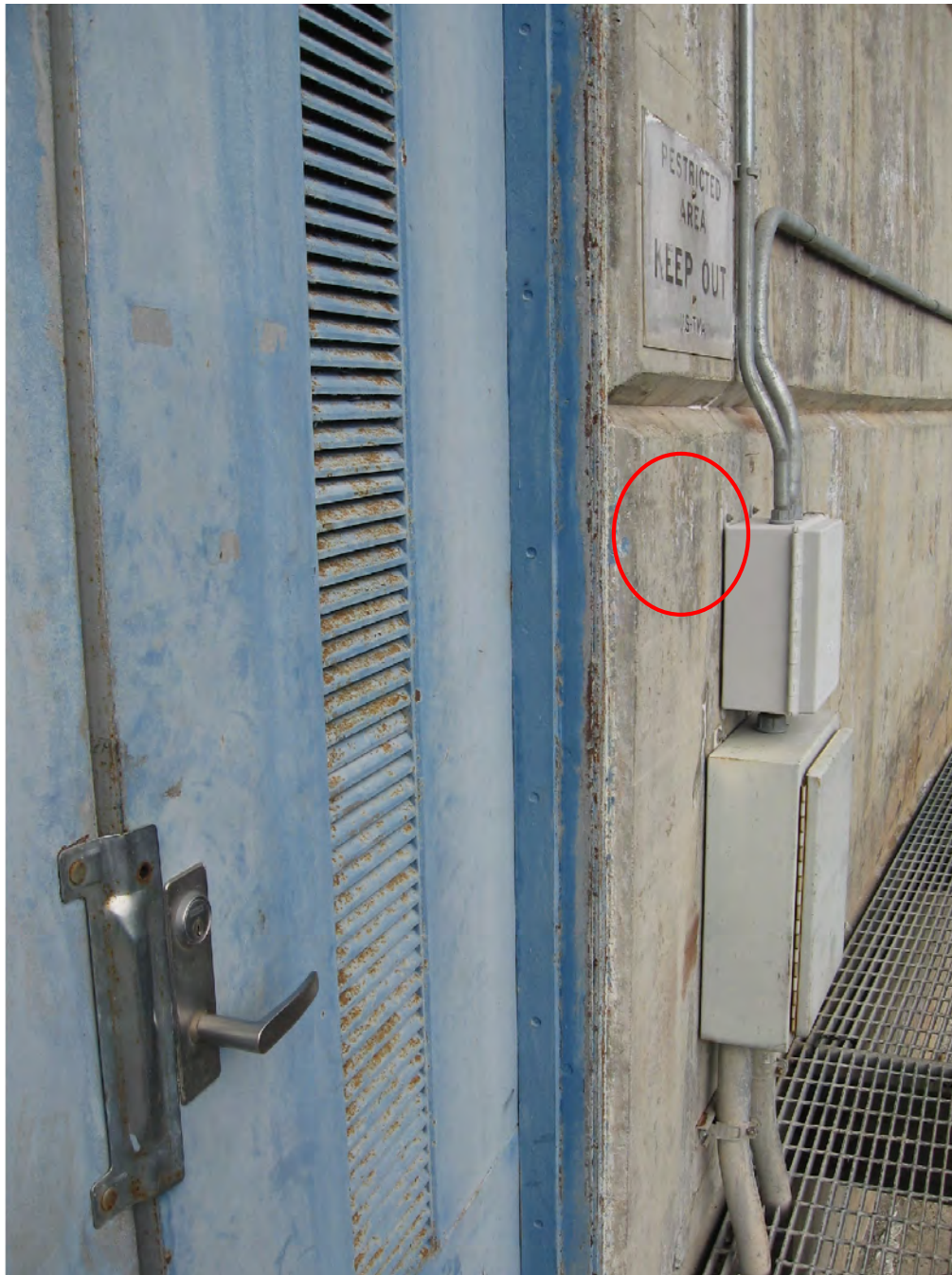
Figure 38: A new card reader will be added to this location circled in red adjacent to the entrance to the east-end Head Gate Gallery door on the south elevation of the dam.
