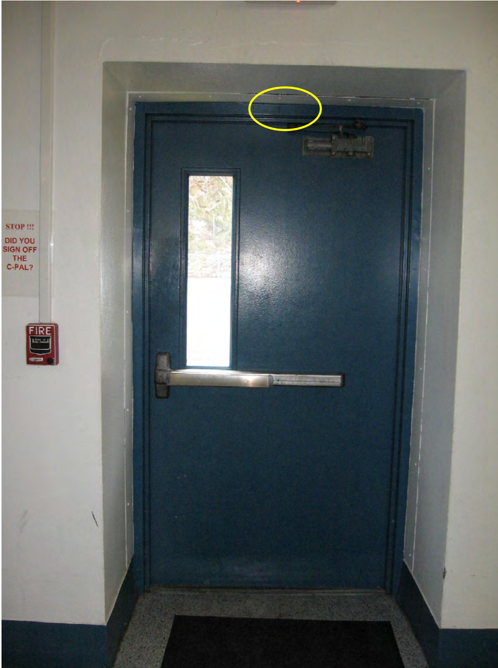
Figure 18: This view is of the interior of the southwest Control Room door and the location of the passive infrared sensor (PIR) is shown as the yellow circle.
